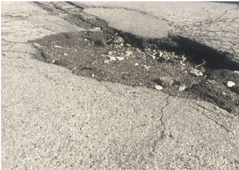
The MASSIVE potholes are a problem for everyone
